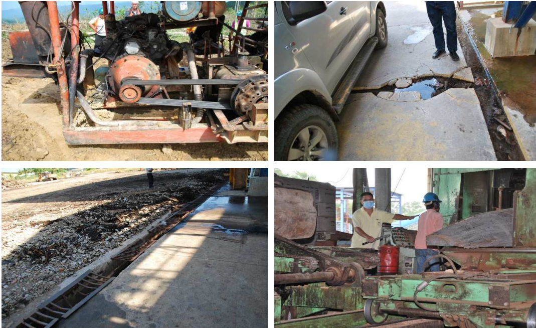
Figure 4 Health and safety issues identified during panel visit.
